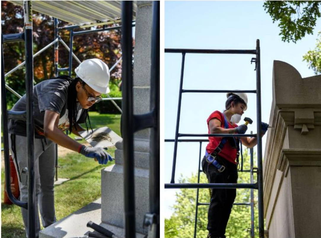
Left, intern Danayris Ramirez, 19, repointed the mortar joints of the Henry Clews mausoleum. Right, intern Stacy Delgado, 22, hammered and chiseled the mortar joints of the Capt. Robert Band mausoleum. PHOTOS: DESIREE RIOS FOR THE WALL STREET JOURNAL
